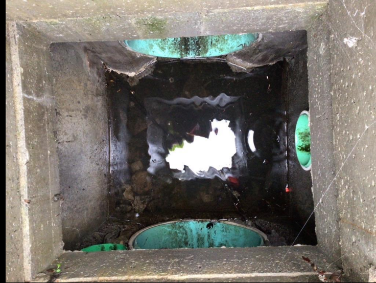
Interior Photo with PVC pipes
