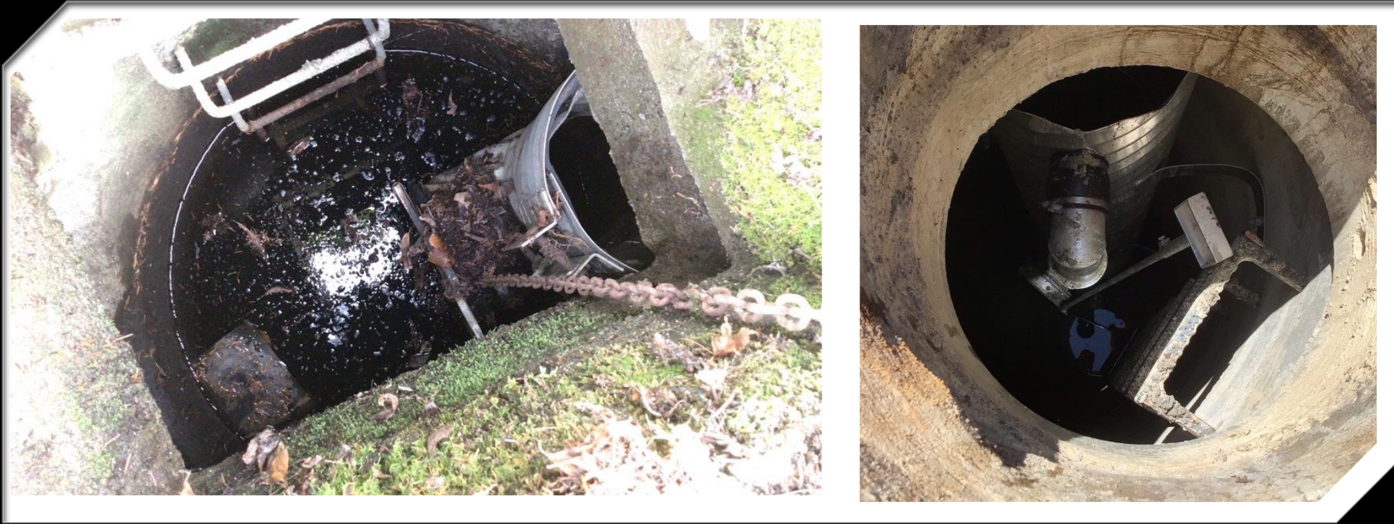
Photos taken from ground level of flow control within a type 2 catch basin.
