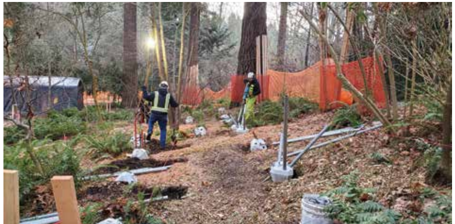
Installing diamond pier foundations for the walkway coming to Kruckeberg Botanic Garden
