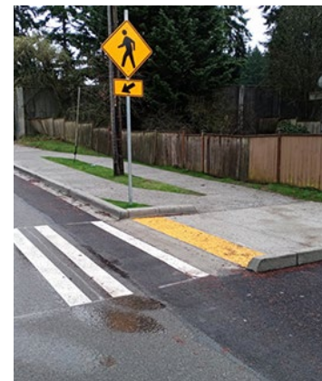
We improved a shared-use path in the Echo Lake neighborhood by installing a new crosswalk and ramps.
