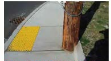
F Category | Most Significant Barrier: Ramp obstructed by pole
