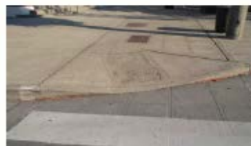
D Category | Significant Barrier No detectable warning present
