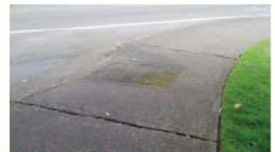
E Category | All elements non-compliant
