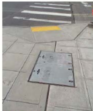
C Category | Moderate Barrier Turning space obstructed by access cover
