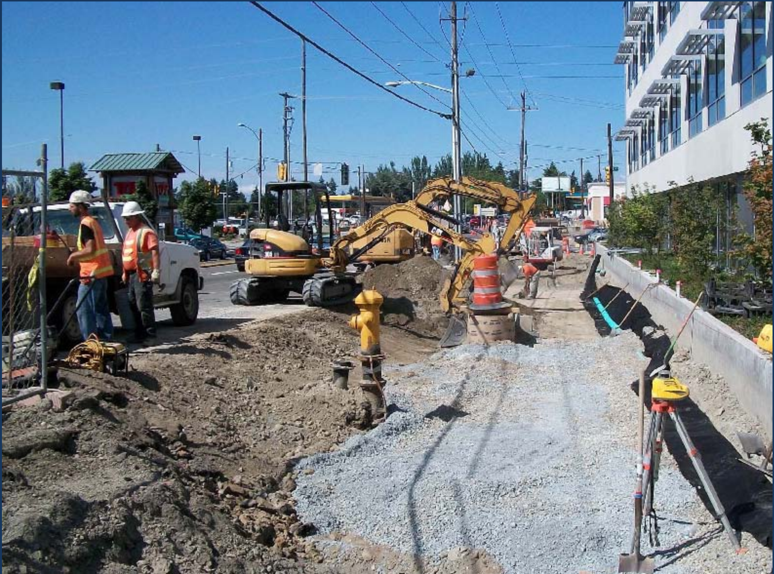
A sub base aggregate is placed in the excavated trench and compacted.
