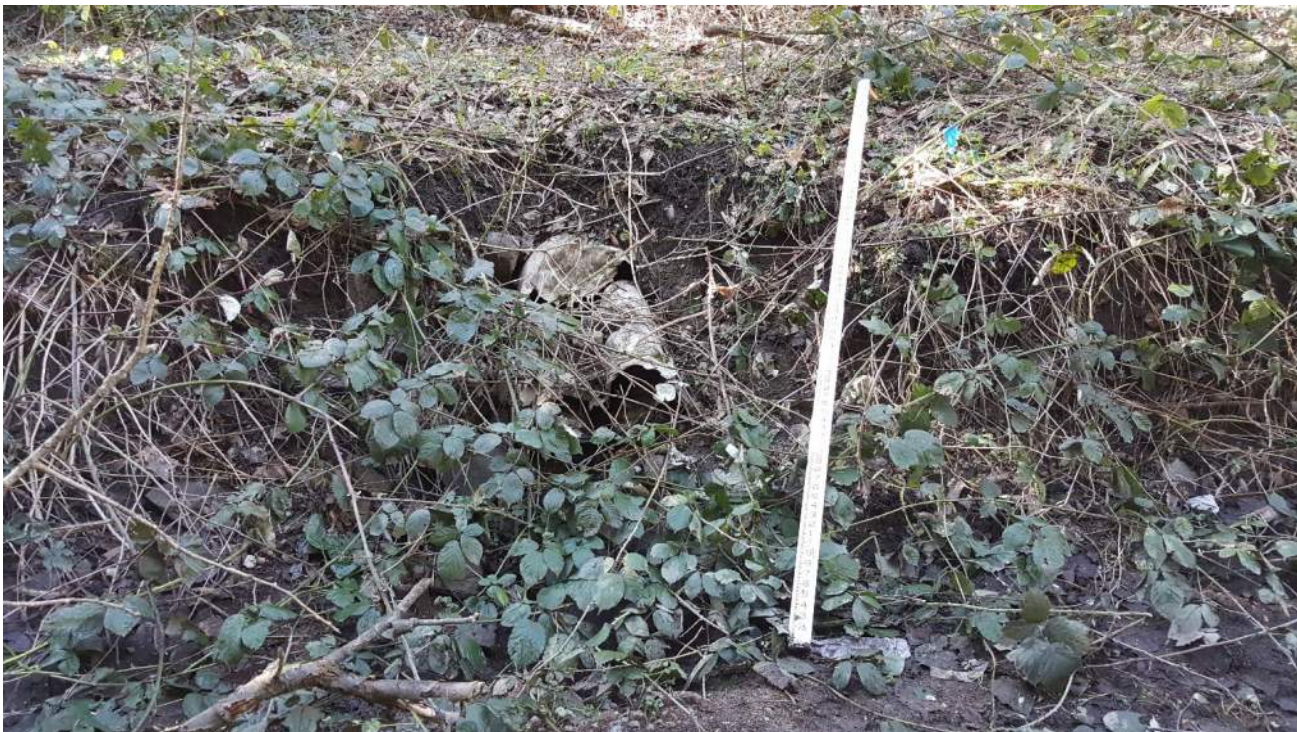
Photo 8. Crushed 18" CMP and bank erosion on the left bank at the bend in the channel.
