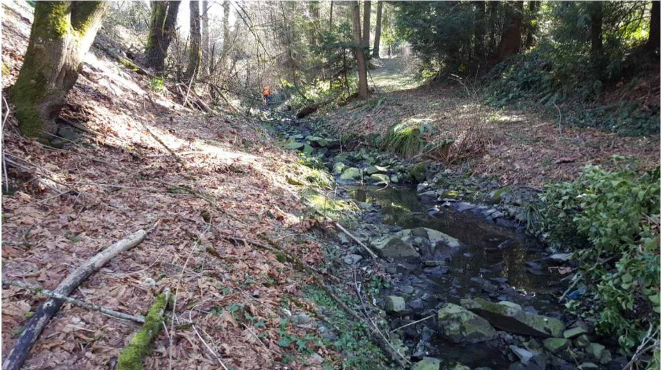
Photo 1. Upstream reach of the South fork of Boeing Creek with riprap armoring, with above ground flow, looking upstream towards the culvert outlet under Greenwood Ave N.
