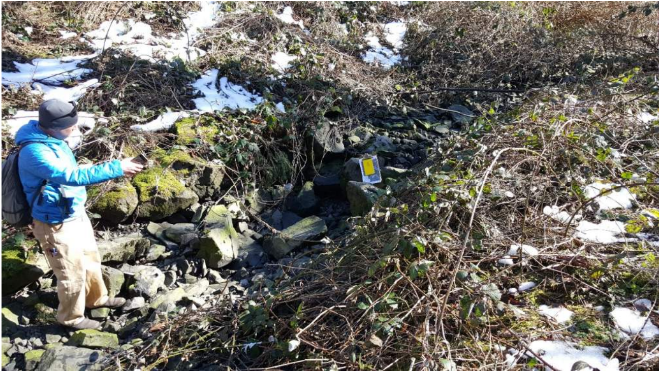
Photo 3. Entrenched channel with rock drop structure near the middle of the project area.
