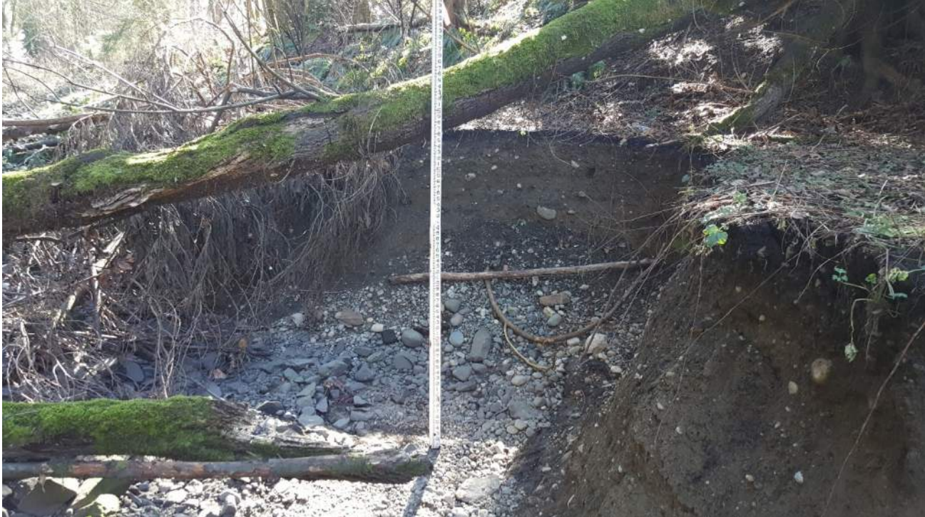
Photo 5. Scour in the left bank of the channel and access road, beneath the tree fallen into the channel.
