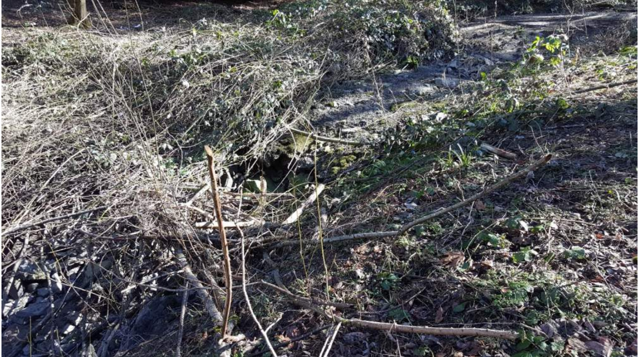
Photo 9. Looking upstream at the gouted riprap grade control structure, upstream of the sediment basin for the M1 Dam.
