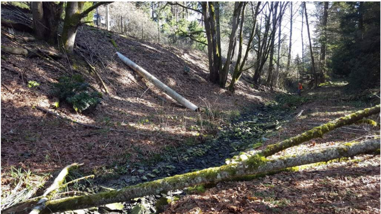
Photo 2. Looking upstream, the maintenance access road abuts the channel on the right side, the exposed 18" CMP is on the left side, and tree have fallen across the access road and channel in the foreground.
