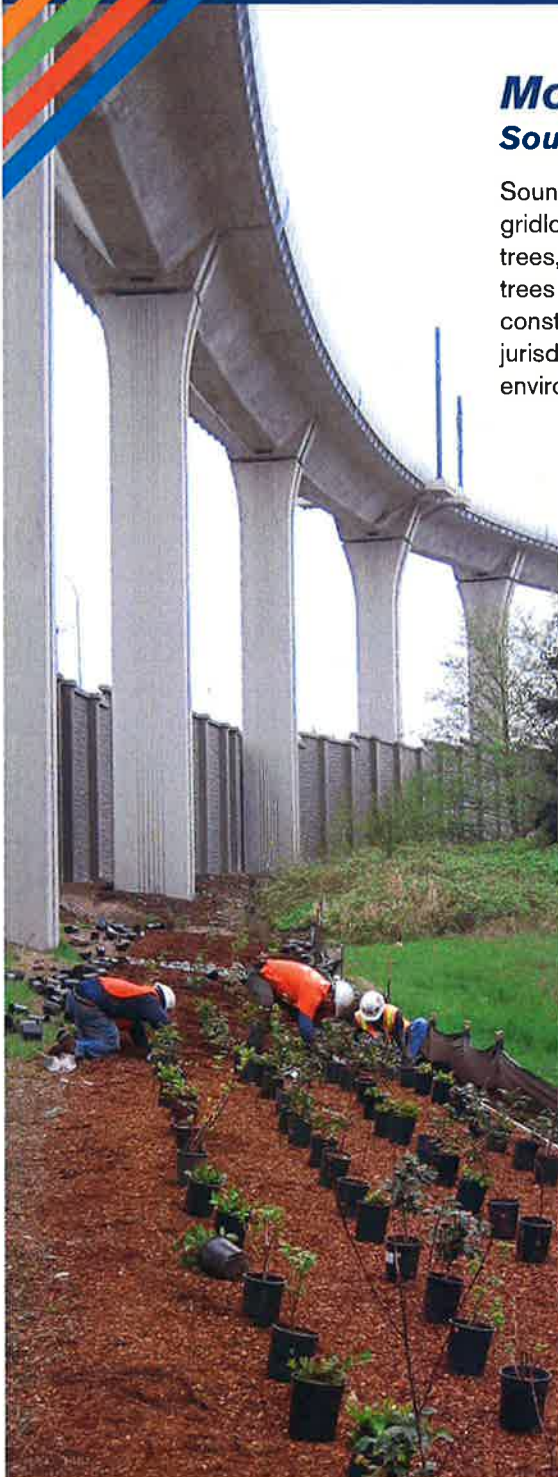
Sound Transit contractors plant one-gallon trees below the light rail guideway in Tukwila. Lynnwood Link will start with 2-5 gallon plantings to better ensure the long-term success of replaced trees.
