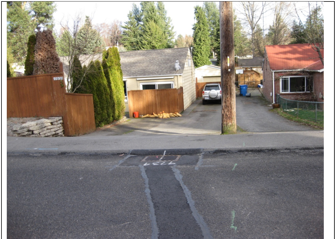
Photo 3: Residence #17030 10th Ave NE, lot#1270, with sandbags. New asphalt patch shows installation of catch basin at gutter flow line. (February 13, 2014)
