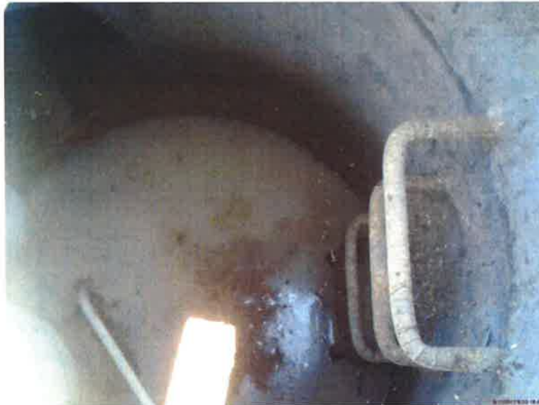
Figure 5-1. Illicit discharge of wet concrete in manhole
