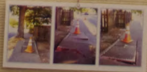
Tree root damage
