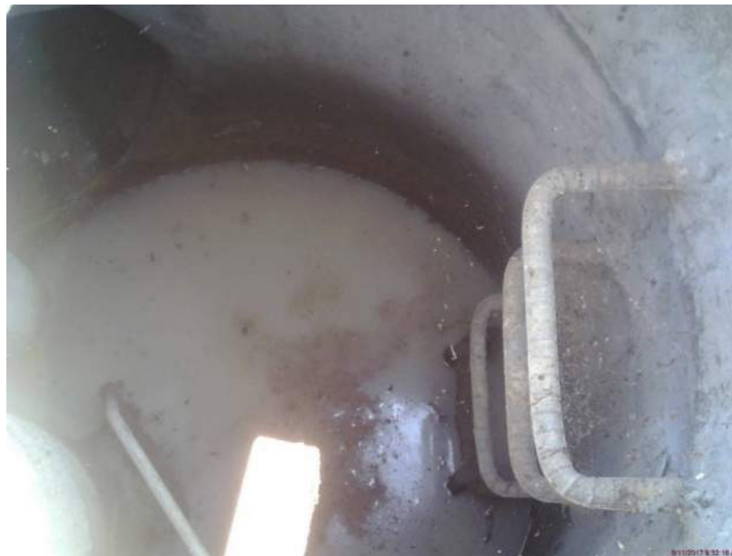
Figure 5-1. Illicit discharge of wet concrete in manhole
