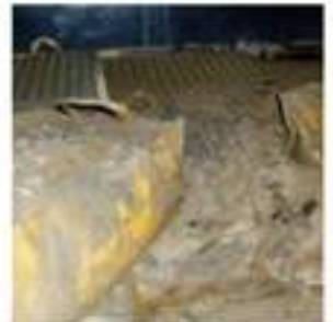
Figure 2. Perlite filter media needs replacement.
