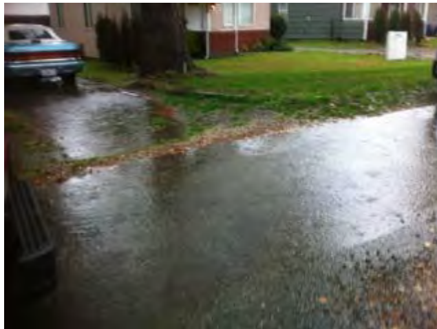
Photo 2 - November 19, 2012 Rain Event Ponding along 148th*
