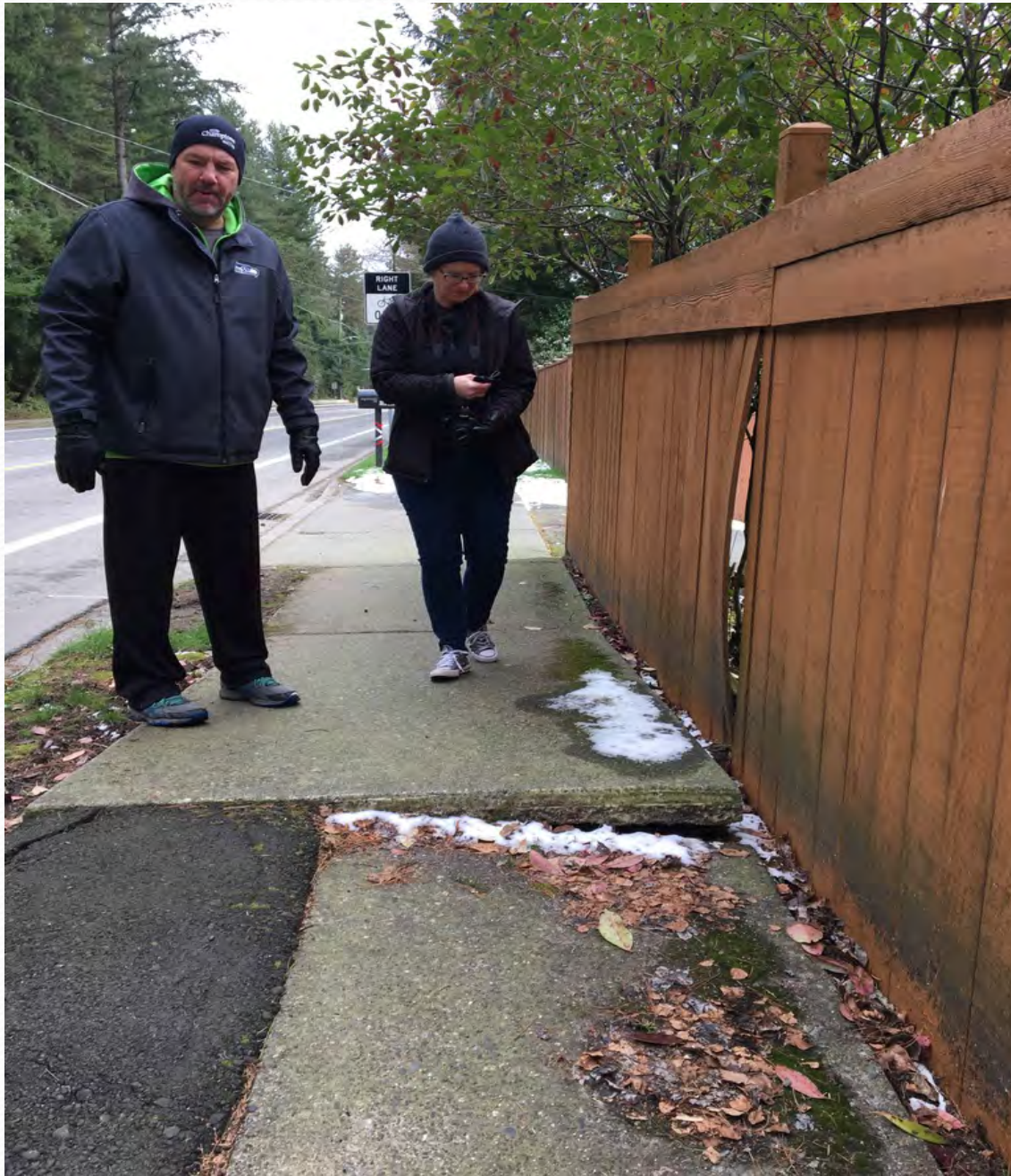
15 th Ave NE – tree root lifts sidewalk panel west side of street, south of NE 165 th St.
