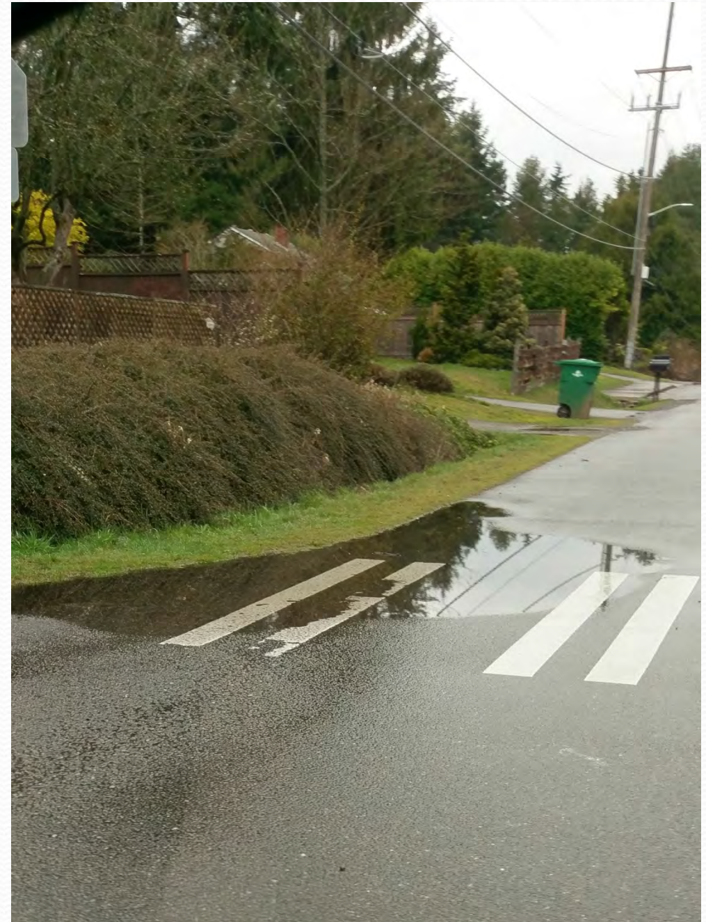
8th Ave NE and NE 170 th – ponding in crosswalk
