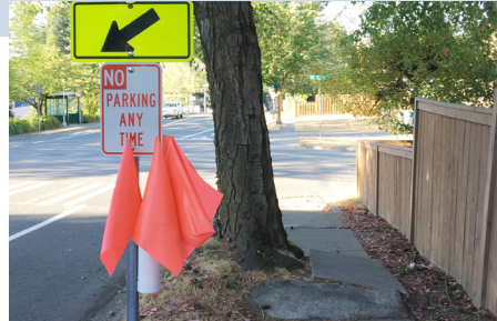
Tree roots lift and crack pavement
