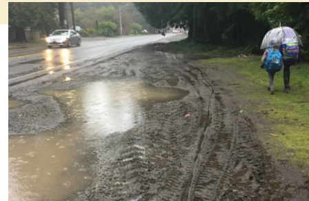
Puddles are obstacles to walking along roadways
