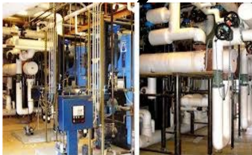
CENTRAL PLANT Plant on roof of building
