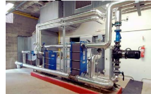
BUILDING CONNECTION Heat Exchanger
