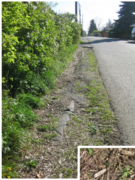
NW 199 th and 21 st Ave NW Broken Pipe
