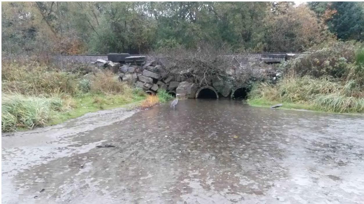
Figure 6. Great Blue Heron Fishing at the Culvert Outlet of Pipers Creek on October 26, 2016.
