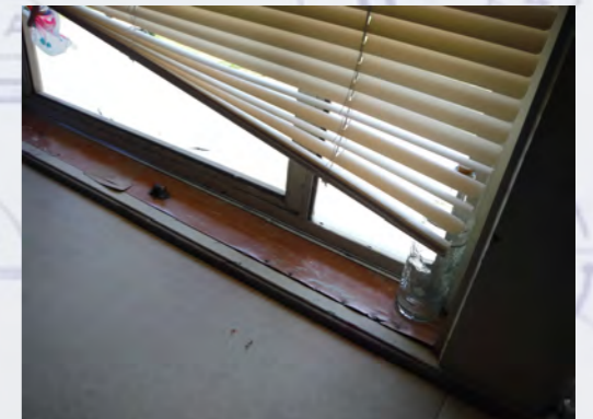
Single glazed, sill rot
