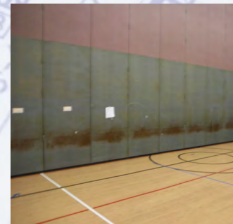
Failing gym partition
