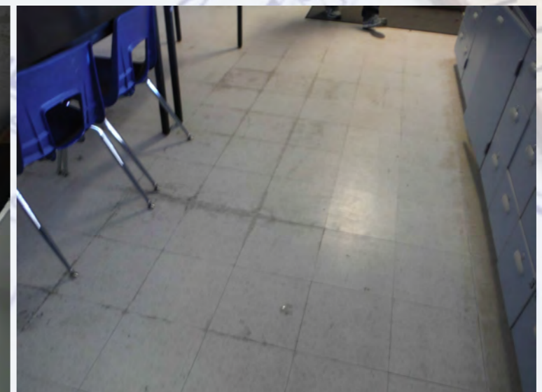
Floors – cracks and surface wear
