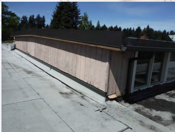
Failing siding and roofing
