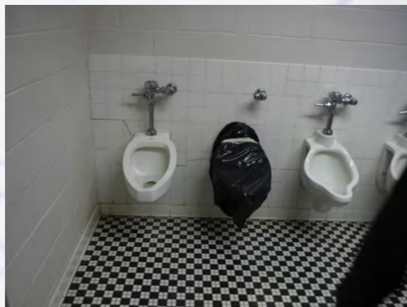
Plumbing & wall cracks
