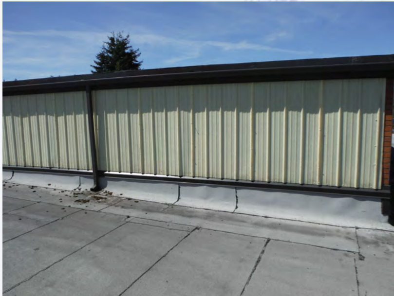
Fiberglass clerestory (natural light) panels
