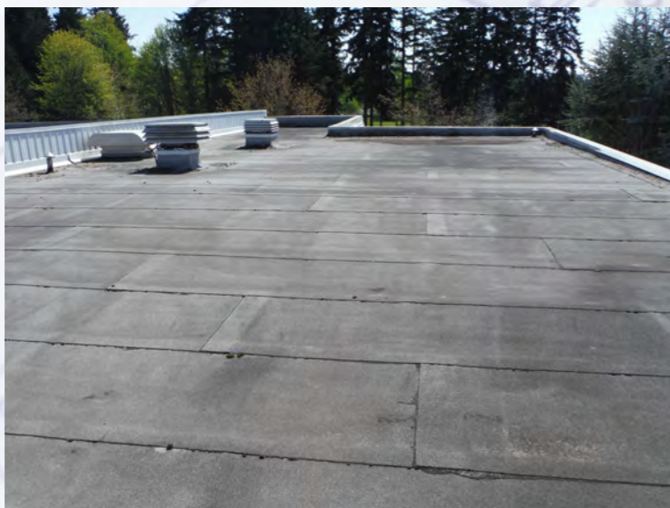
Roofing – surface wearing out
