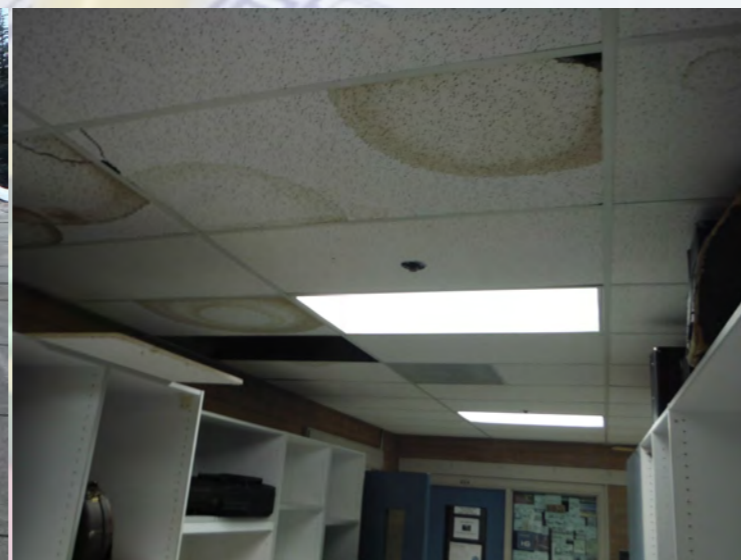
Ceilings – water stains
