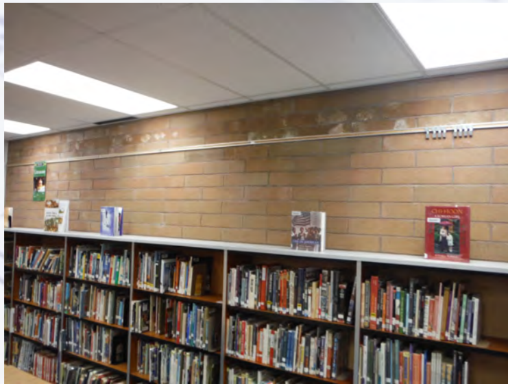
Masonry walls – poor insulation
