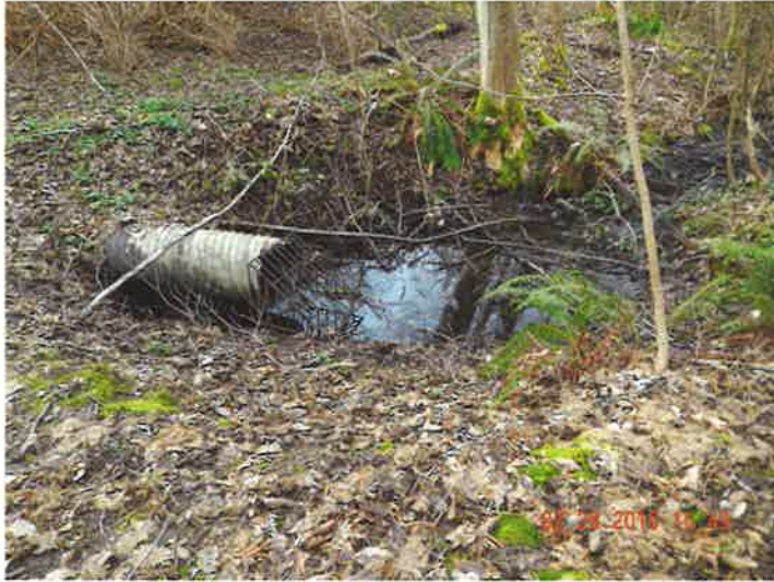
P17 tributary into pipe under road and south to restoraitn area.jpg
