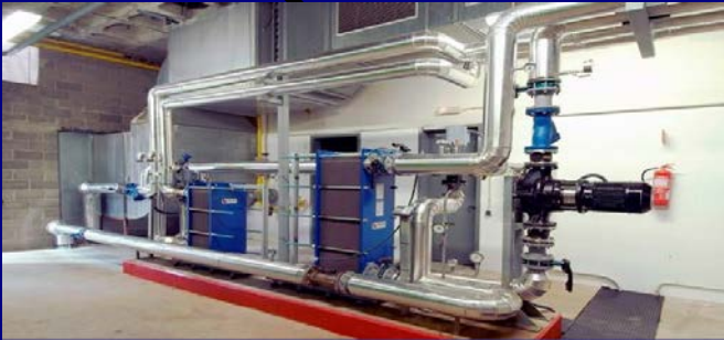
BUILDING CONNECTION Heat Exchanger
