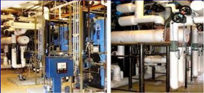
CENTRAL PLANT Plant on roof of building
