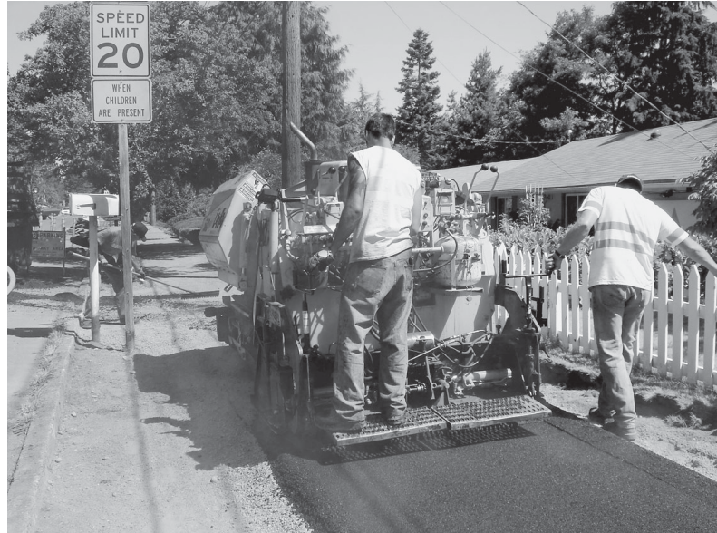
The asphalt pathway being installed along the east side of 10th Avenue NE (shown both above and below) will be complete before school starts in September.
