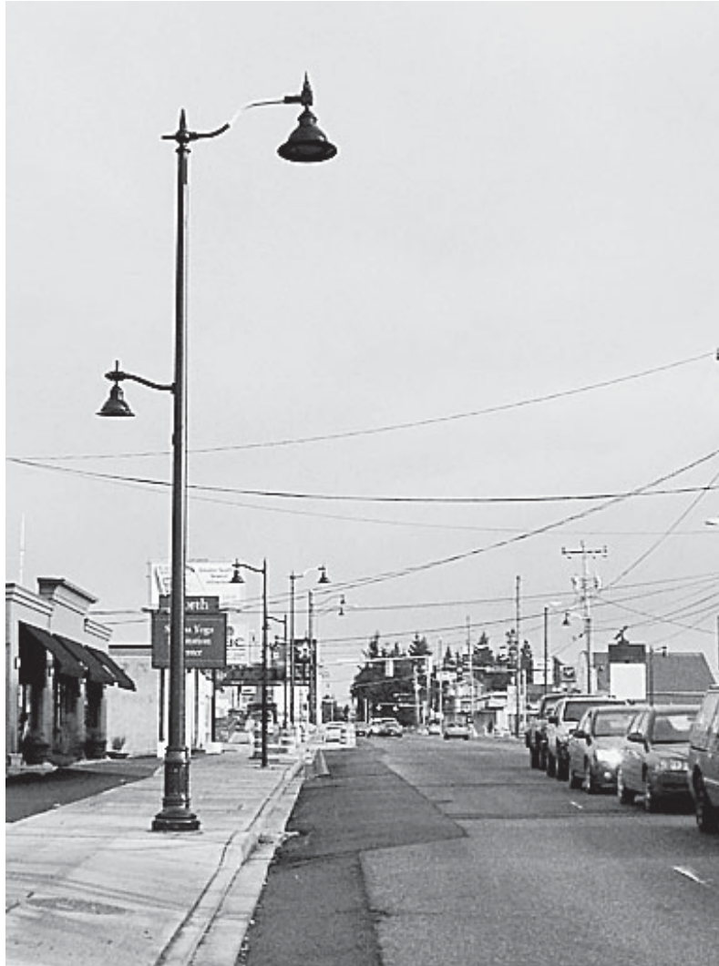
New light and signal poles have been installed along 15th Avenue Northeast as the North City Project nears the last two months of construction.
