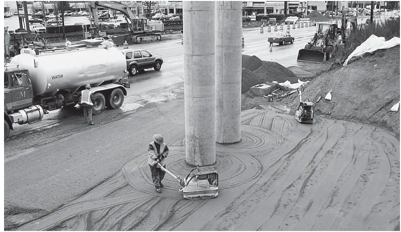
Crews compact fill around the base of the columns that will support the Aurora Interurban Trail Bridge on the east side of Aurora.
