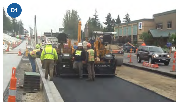
D1. Paving the first lift of the future southbound business access and transit lane
