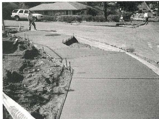
The Serpentine Drainage Improvement Project included new sidewalks, curb and gutter along NE 175th St. as well as installation of storm drainage pipe and a new pump station.
