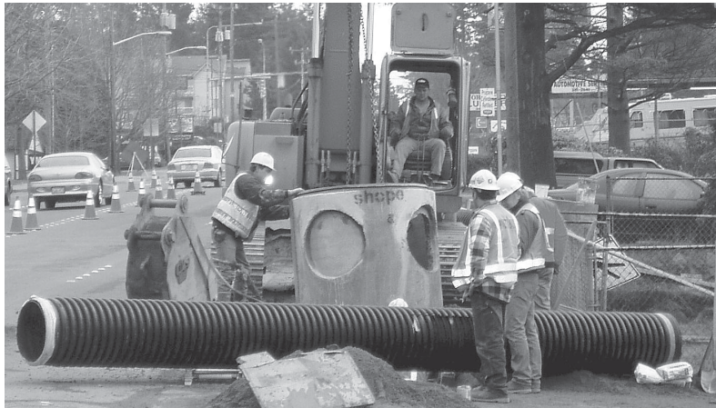
Part of the work for the Serpentine Place Drainage Improvements included replacing a catch basin on N. 175 th St.
