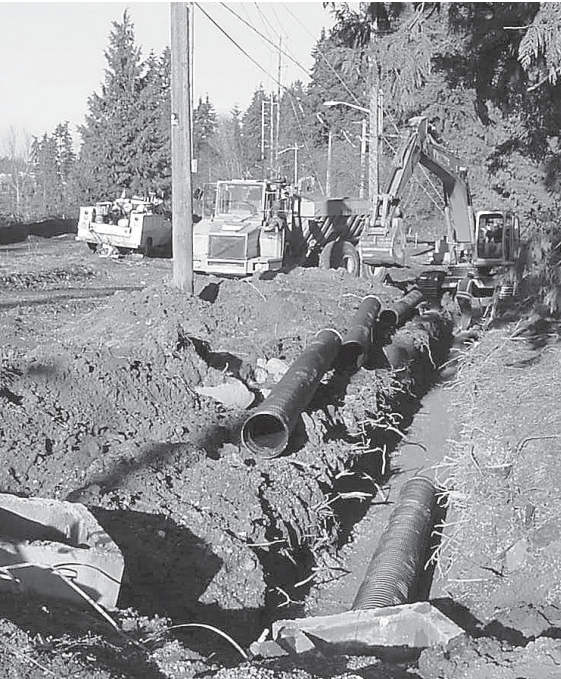
During the second week of February, crews worked on the drainage along the Interurban Trail near N. 192nd St.
