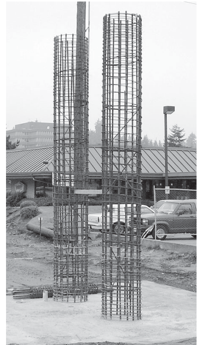
Crews built the rebar forms for one of the piers for the N. 155th St. Bridge.
