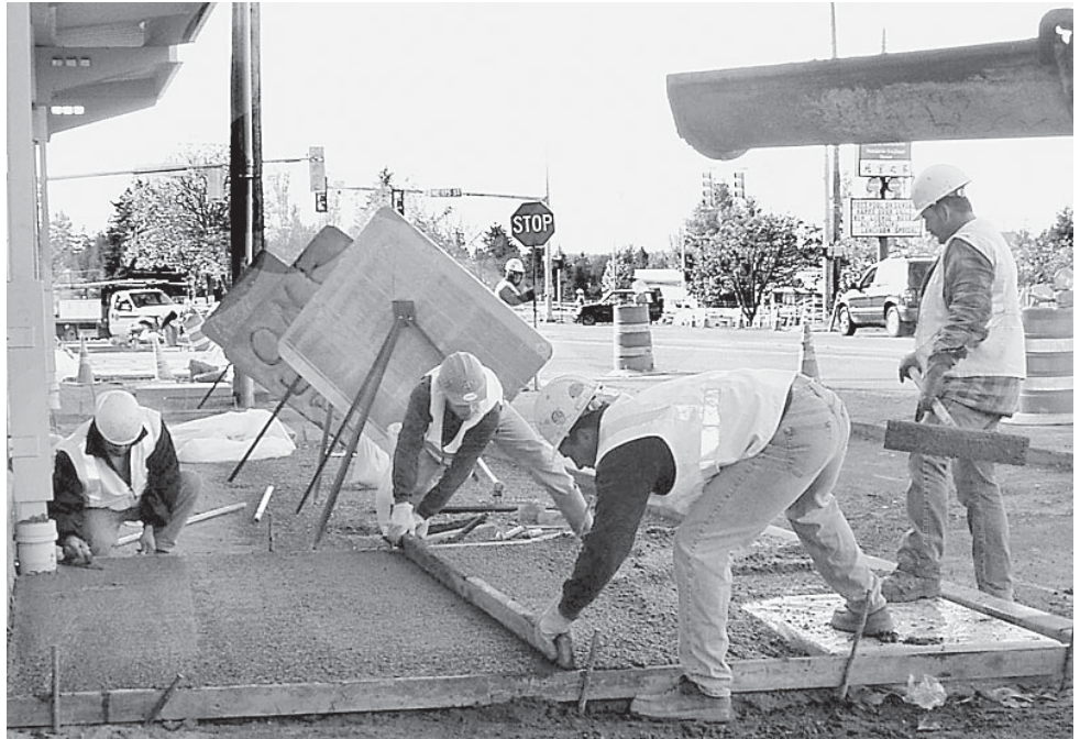
Pouring sidewalks has been one of the major focuses of the North City Project in the past few months.
