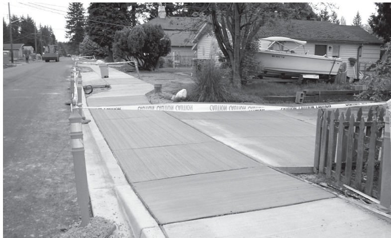
The curbs, gutters and sidewalks along 3rd Ave. NW have been completed and landscaping is the next step for construction of the 3rd Ave. NW Drainage Improvement Project.
