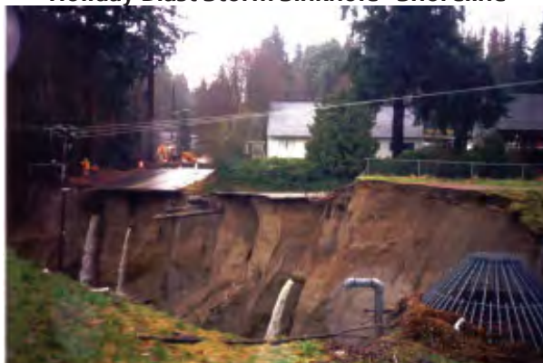
Figure NEA-2 Holiday Blast Storm Sinkhole - Shoreline
