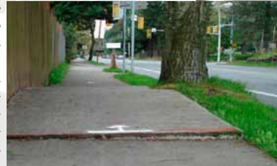
Sidewalk damage caused by tree roots
