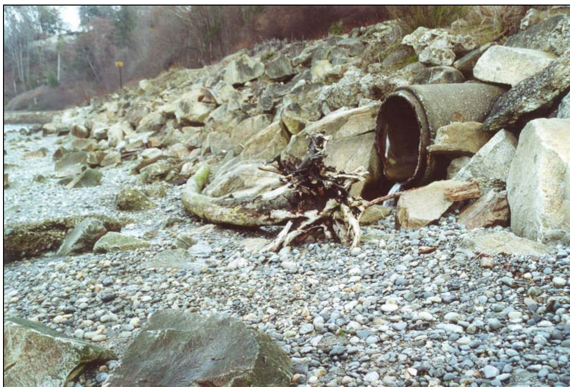
Photo 19. Unnamed Creek Culvert under BNSF Railroad Tracks in the Middle Puget Sound Basins
