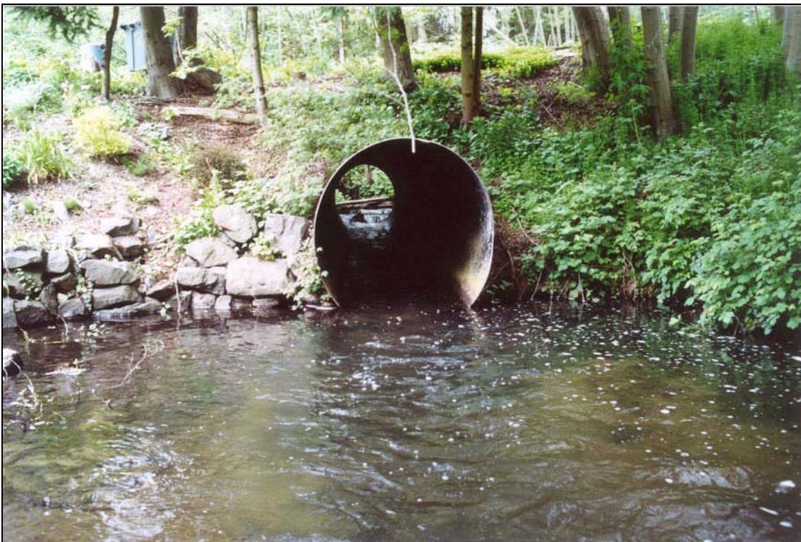
Photo 12. Culvert Under Forest Park Drive on McAleer Creek; Blockage at Upper End of Pipe
