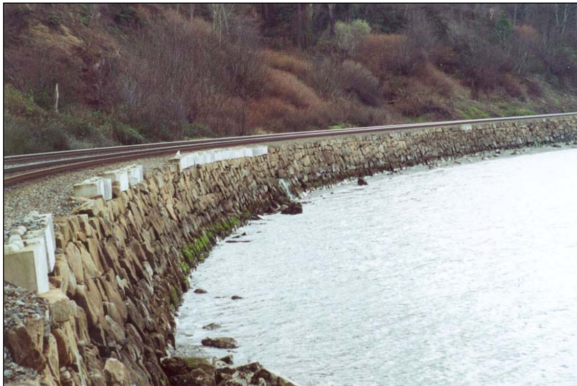
Photo 18. Unnamed Creek Culvert under BNSF Railroad Tracks in the Middle Puget Sound Basins
