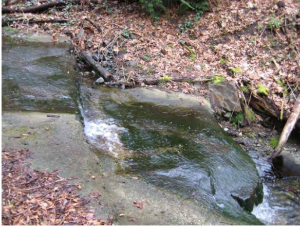
Photo 3. Concrete poured over sanitary sewer line in Storm Creek – likely fish passage barrier
