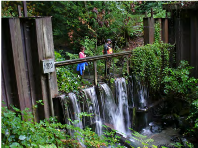
Photo 15. Seattle Golf and Country Club sheet pile dam (upstream limit of anadromous fish access in Boeing Creek
