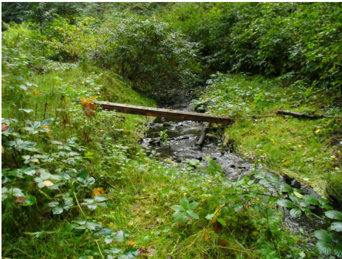
Photo 10. Sediment terrace remaining from 1997 washout
